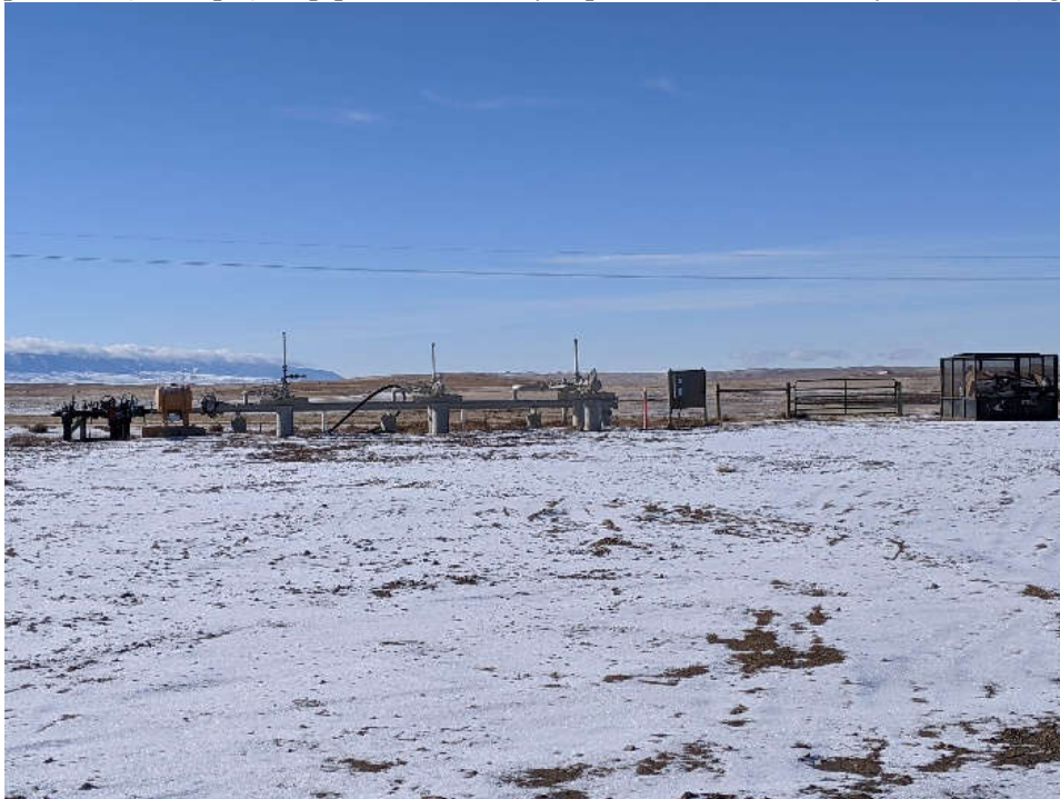
Figure A-4: The Pipeco owned source gas pipeline header
