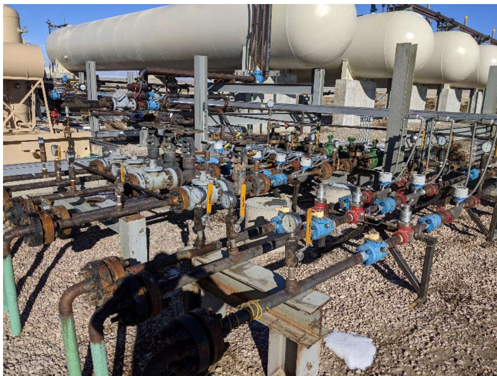
Figure A-7: The injection well manifold (working pressure 4,000 psi), coming off the discharge line of the second stage compressor
