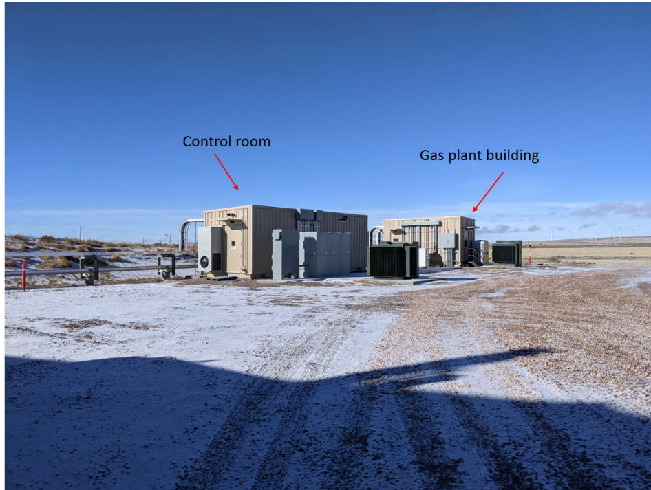
Figure A-5: The gas plant and control room buildings
