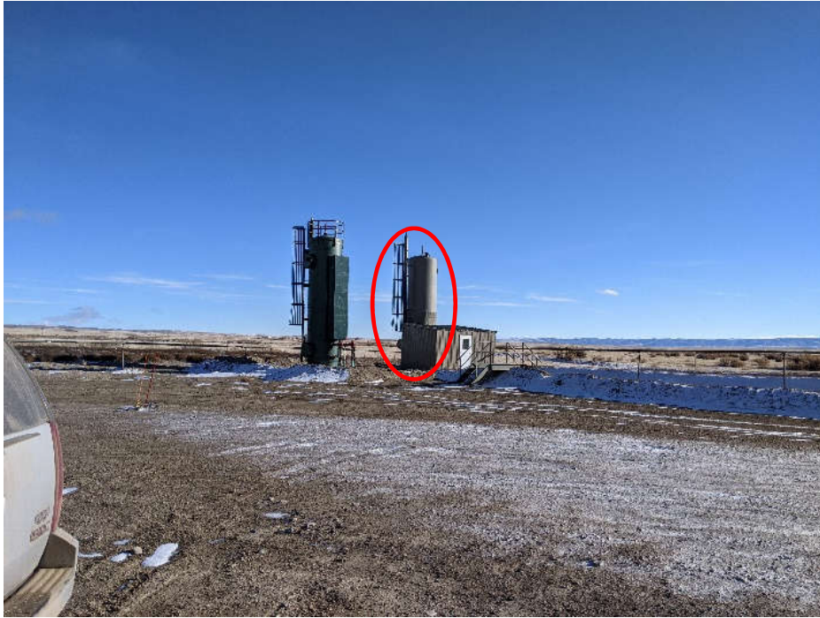
Figure A-2: Example of a single well battery heater-treater unit, circled in red
