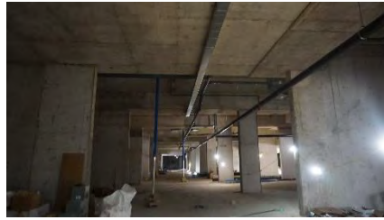
P1 – Sprinkler main and MUA ductwork
